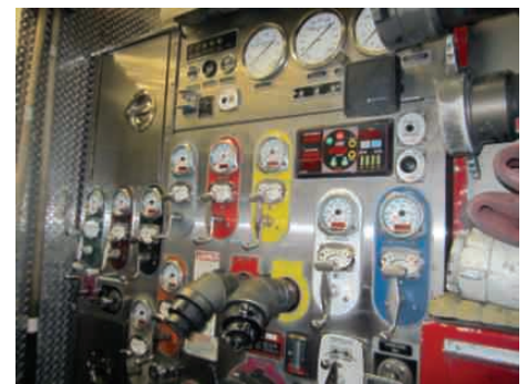
Controls for pump on Engine 8.
